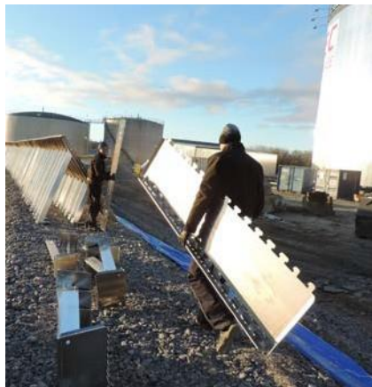
Photo showing installation of the H180 barrier. Simple to carry and handle, only 27.5kg per section.
