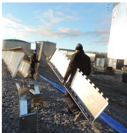
Photo showing installation of the H150 barrier. Simple to carry and handle, only 25 kg per section.
